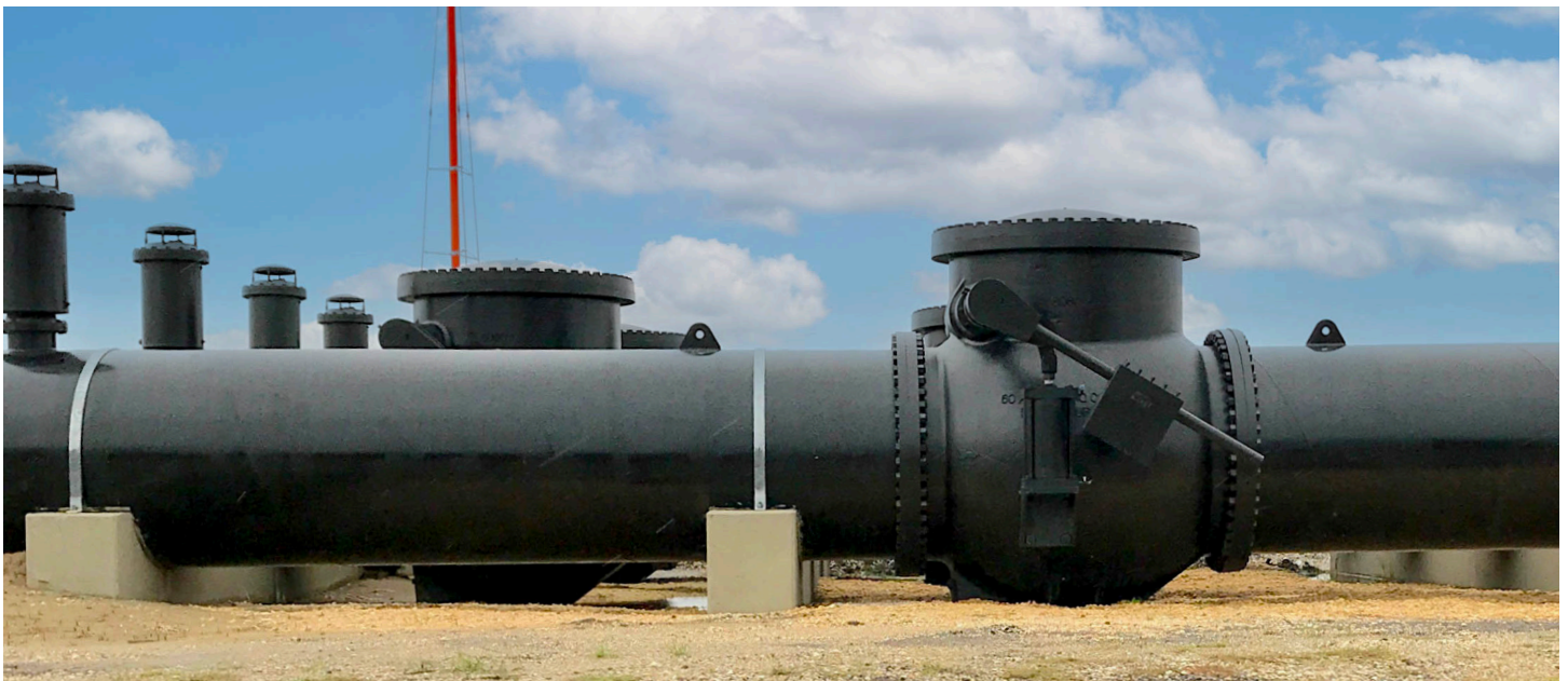
Four 60" APCO CVS Swing Check Valves and ASV Air Vacuum valves are part of a pump station that directs stormwater away from the Louis Armstrong New Orleans Airport to protect against flooding damage during tropical storms.
