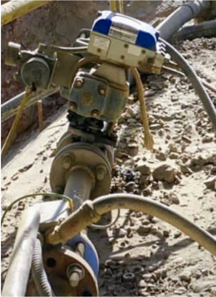
Field installation of 2" RCV for raffinate control
